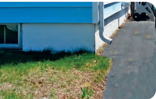
Roof runoff directed onto this driveway flows into the street and may be sending pollutants to a nearby waterbody.
